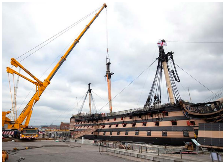
A £35 million conservation project to renovate HMS Victory, including replacing rotting planks, has been announced on the 100th anniversary of the warship being brought into dry dock.
