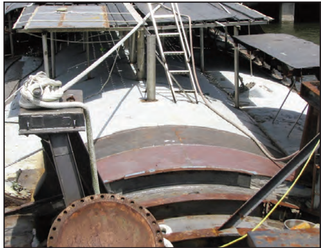
Above: The exposed pressure hull of Clamagore, definitely a rare sight! Photo by John Makara.
