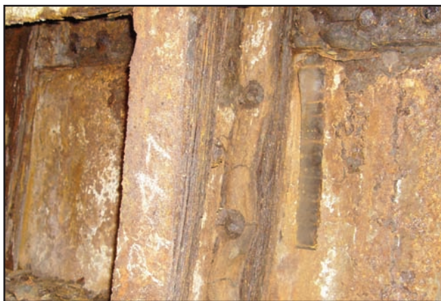
Above: An example of extensive corrosion damage due to prolonged damp conditions.
