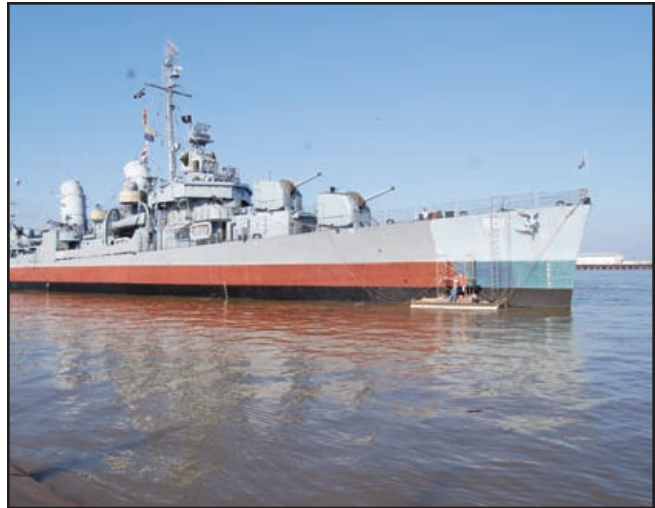
Above: Staff and volunteers of the USS Kidd painting the hull of their ship in June 2009 from their recently donated new paint raft. Photo by Bob Holt.
