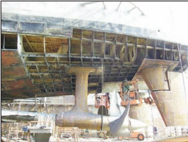
Above: View of the stern with old hull plating removed. Photo by Joe Lombardi
