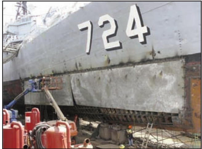
Above: "Off with the old..." Workers remove the damaged hull plating from Laffey's starboard side.
