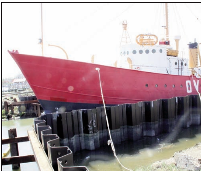
Above: Portside view of Overfalls shows construction in foreground of new slip that was completed in June 2010.
