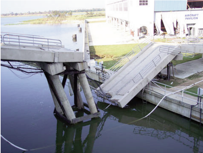
Above: Damage to the ramps leading up to the ship caused by Hurricane Katrina.
