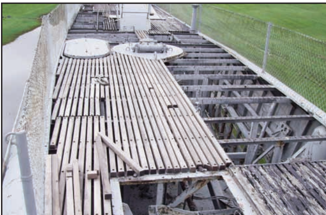
Above: The current deck situation on Batfish showing the extreme amount of work need to restore the ship.
